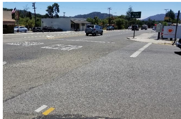
Figure 19: Incomplete limit lines and missing pedestrian crosswalk
