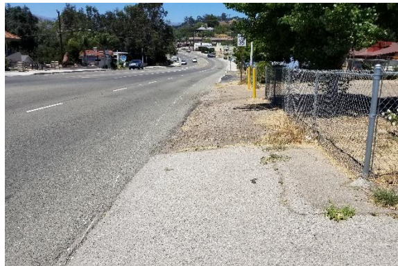
Figure 7: Side of Highway 33 inconsistency with asphalt and natural ground.
